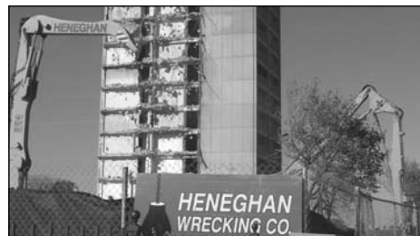
Private contractors tearing down public housing units at Cabrini Green Projects in Chicago.
